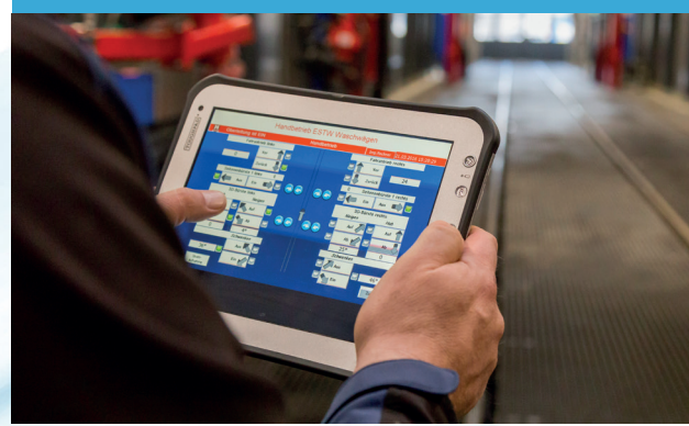
▲ Wash system for long-distance/passenger trains (above) Control panel (below)
