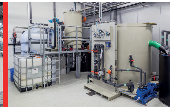
◀ From left to right: Tram washing system Cable drag Bioturbo
