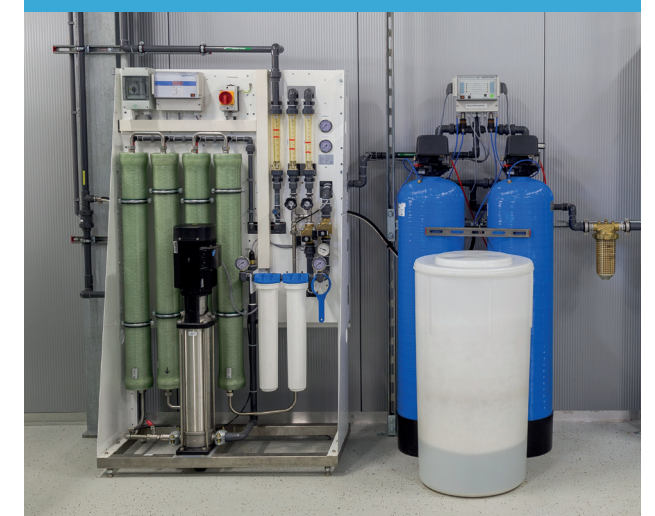
▲ Commercial vehicle wash system (above) Osmosis system (below)
